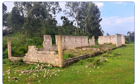
Figure 1. Kindergarten site, dilapidated before construction completed. Photo by the author.
